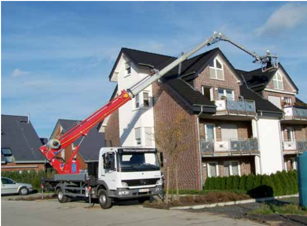
Image 0 Böcker cranes can be converted into work platforms in just a few steps. Particularly high safety standards apply to these.
