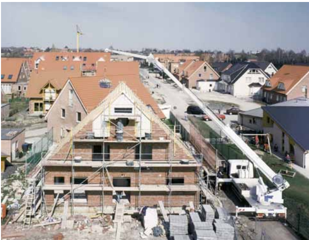
Image 1 The support system is variable and can be adjusted to the circumstances onsite. This creates completely asymmetrical operating ranges which are calculated and monitored by sophisticated sensor technology.
